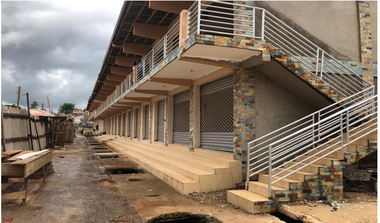
3NO.165-Units Lockable Stores substantially from Internally-Generated Fund (IGF) under construction by the West Akim Municipal Assembly at the Asamankese main Lorry Park.
